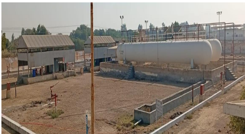
LPG Air Mix Plant Kot Ghulam Muhammad, District Mirpur Khas, Sindh
